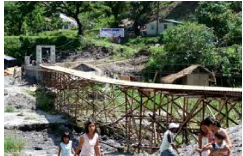
Engineers work on the construction of a hanging footbridge as part of an ASEAN disaster response exercise in Sapang Bato, Philippines (credit: DFAT).
